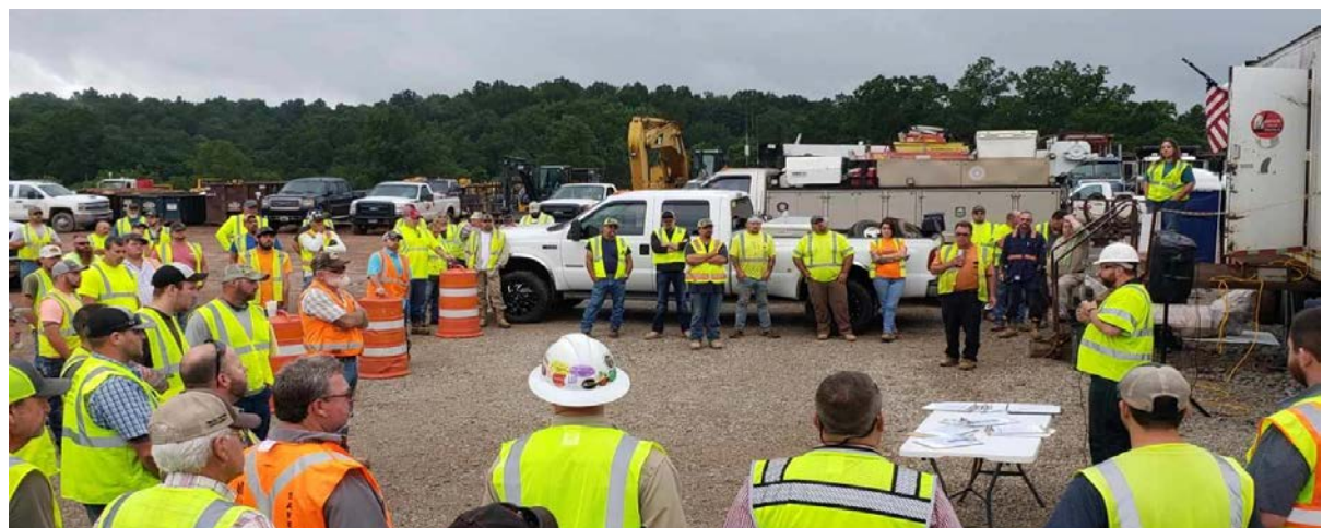
APLC hosted Anthony Miliam, OSHA Compliance Assistance Specialist, on our MXP Project on June 17, 2019. Mr. Miliam spoke in depth regarding Trench Safety, challenges and mitigation means for trench safety.
